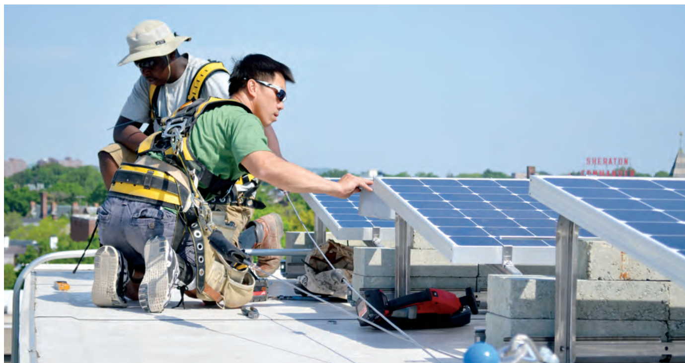
UCS’s Cambridge headquarters updated its two-decade-old photovoltaic array with a larger, more efficient system that generates six times more clean electricity.
